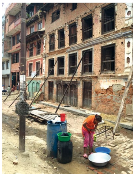
Walls of houses damaged by earthquakes are provisionally stabilized by supporting pillars. (Photo: Bijan Khazai)
