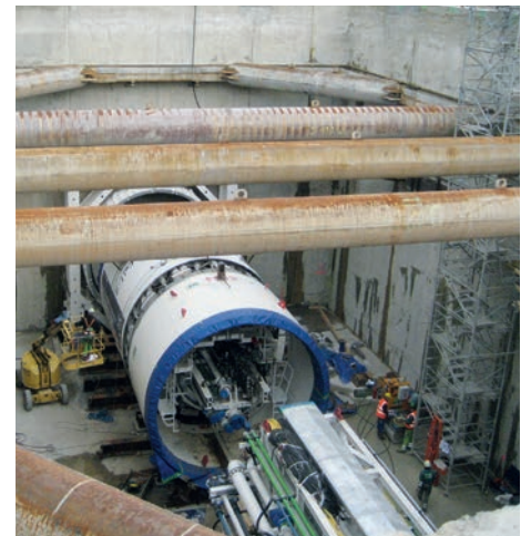
Assembly of the tunnel boring machine in the DESY starting shaft in Hamburg, 2010. (Photo: P. Kudella, KIT)
