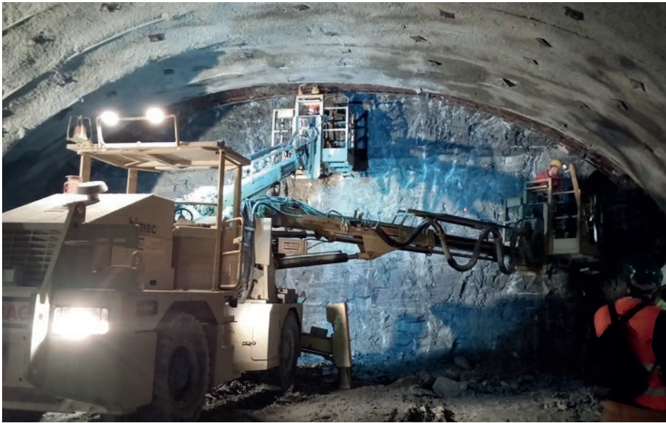
Drilling blast holes to advance the roof section of the Brenner Base Tunnel in 2015. (Photo: P. Kudella, KIT)
